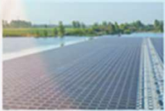
4.2MW floating solar farm in Shandong China
