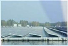
5MW floating solar farm in Shandong China
