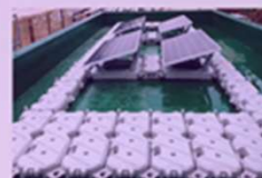
1.48KW floating solar farm on waste pond in Jiangsu China
