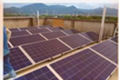
800KW rooftop solar farm in China
