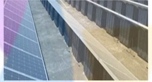
3MW roof system in Australia
